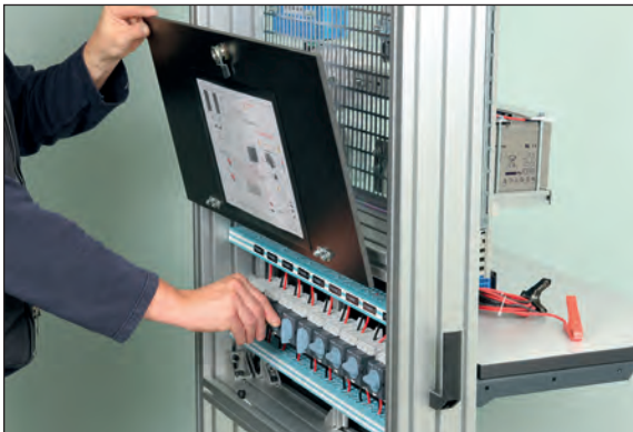
Flap for access to the switches
